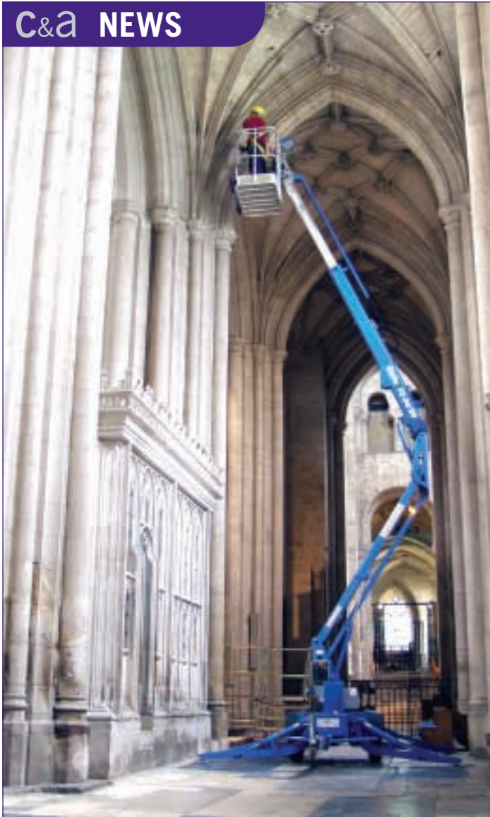
HAMPSHIRE PLANT recently supplied Winchester cathedral with this 12.36 metre Genie TZ-34/20 trailer mounted boom to help with re-wiring work for the building's sound system. ■
