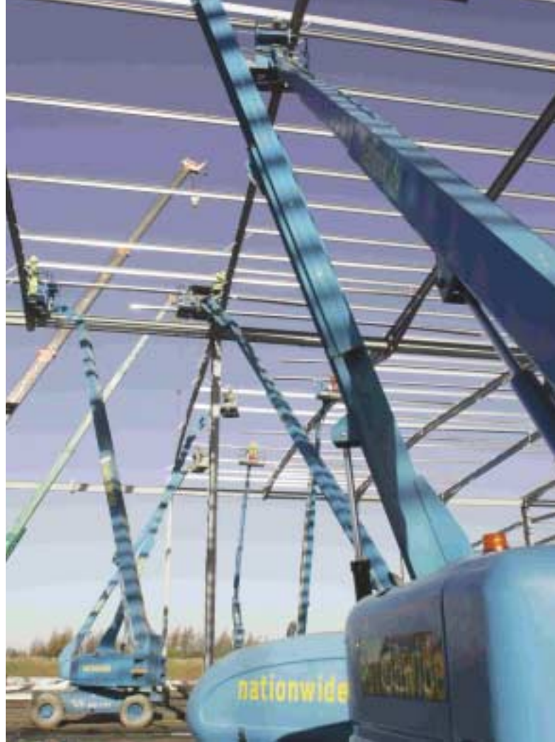
Nationwide Access supplied 14 straight booms to erect 1,400 tonnes of steelwork on the 870,000 Sq metres Magan Park distribution centre in Lutterworth.
