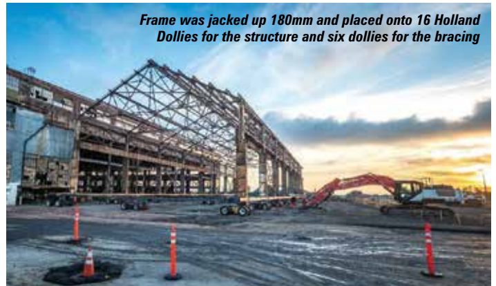
The 175 tonne steel building frame was moved almost 40 metres as part of the Pier 70 regeneration project in San Francisco
