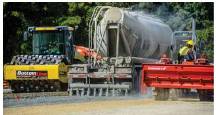
Mammoet's 'Enviro-Mat' creates a strong and durable surface that can increase the load bearing capacity of unstable soils by up to 50 tonnes per square metre
