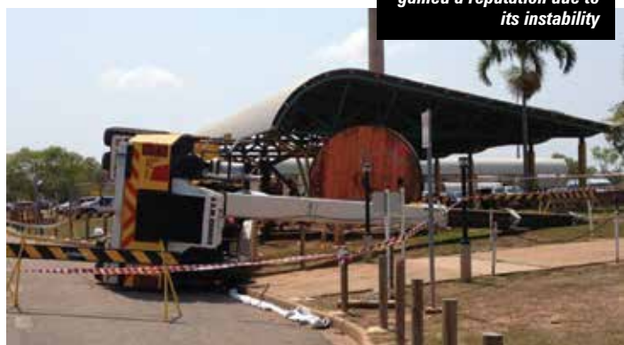
The articulated crane has gained a reputation due to its instability
