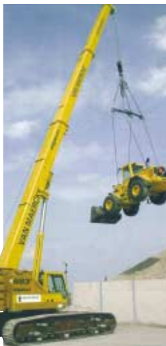
An 80 tonne Heavy duty Sennebogen 683 HD telescopic crawler with 42m boom, owned by Van Marercke of Belgium.
