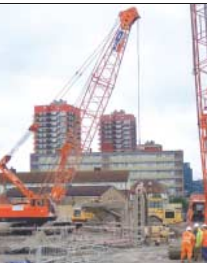
The IHI DCH900, equipped with a heavy grab, is excavating the diaphragm walls to 30 metres.
