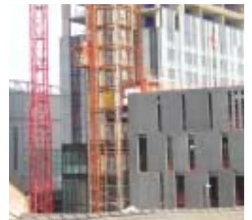
The use of the tower saves space and simplifies logistics.
