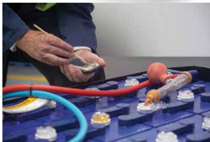
A heavy-duty battery discharge meter.
