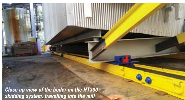
The boilers had to be skidded into the mill under a pipe gallery and between two structures, with just inches to spare on all sides
