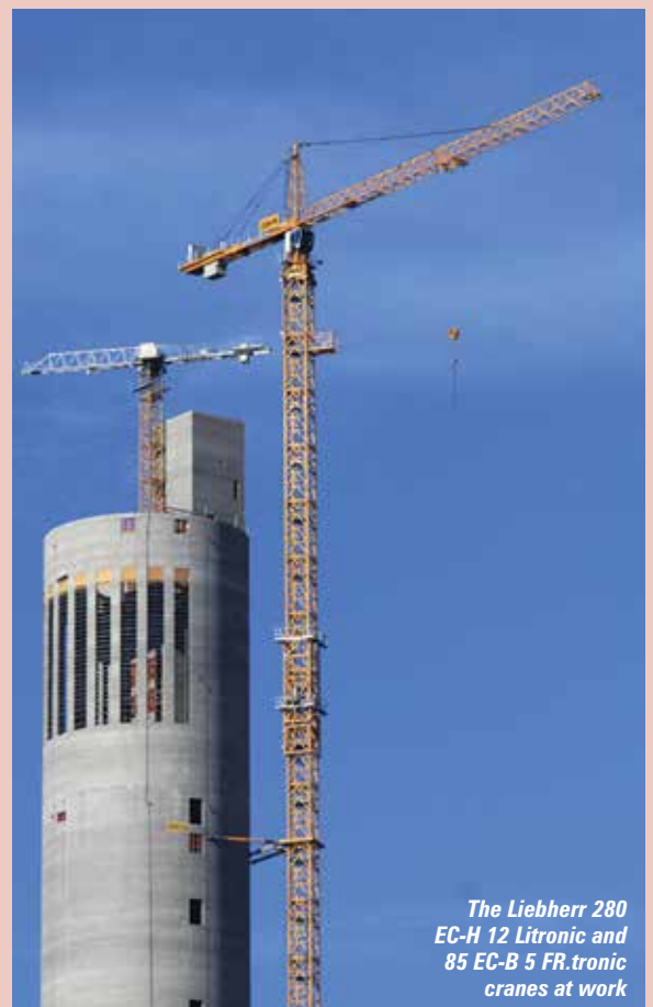
Two Liebherr tower cranes working on the construction of the elevator test tower in Rottweil
