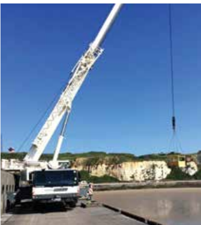
Southern Cranes making full use of the VarioBase technology at Newhaven Port.
