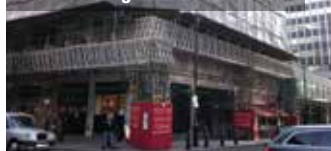
X Beams are used to support full scaffold where pavements won't take the weight
