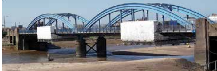
Steel repairs are carried out then blasted and painted with a containment platform which moves to allow river traffic through
