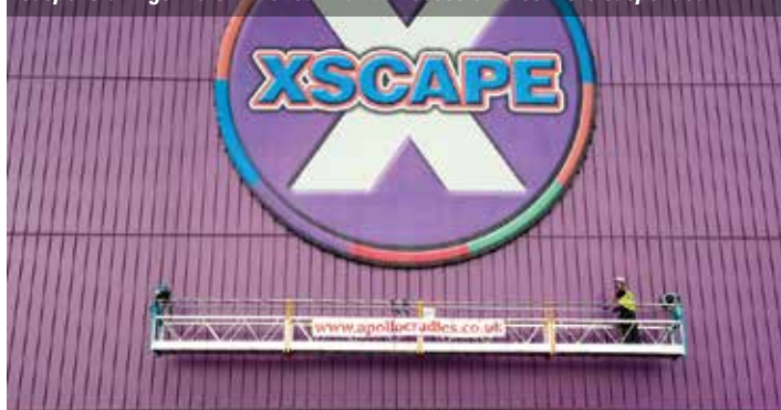
The Xscape Yorkshire building required the external elevations to be covered with cladding and sheeting. For this task, suspended cradles were chosen as the best method. Utilising the I-beam framework of the building, suspension rigs were attached and the access cradles were suspended
