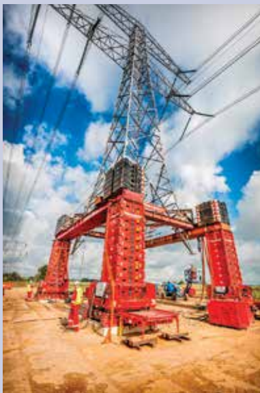
Mammoet has completed the first ever lift of a 'live' high voltage pylon. The 380kV structure was raised in-situ by four metres, while maintaining the power supply.
