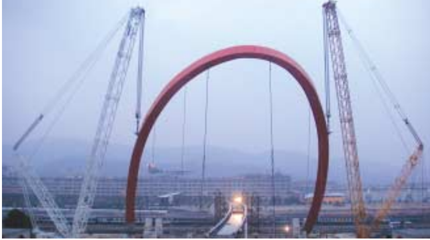
Sarens installed the 524 ton, 64m high by 46m wide Olympic Arch for the Winter Games in Italy. The arch, fixed by two hinges to its foundation, was lifted to 85° by 500 and 600 tonne crawler cranes. Four 185 tonne strandjacks then rotated the arch to 100°, where the cranes helped install the arch at its final angle of 114°
