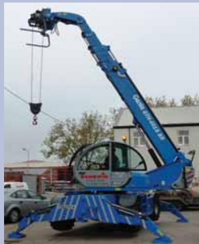
The telehandler is used to unloaded components, carry lift and position them ready for fixing at a height of 17 metres.
