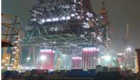
ALE successfully jacked a 42,780 tonne load thought to be the heaviest load lifted in a jack-up
