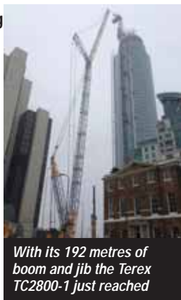
St Georges - the tower crane before the crash
