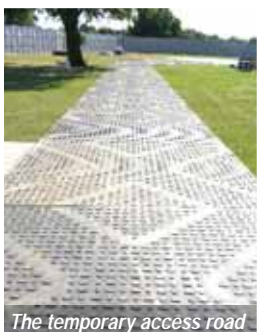
The crane sat its regular steel mats on top of the Tufftrak mats
