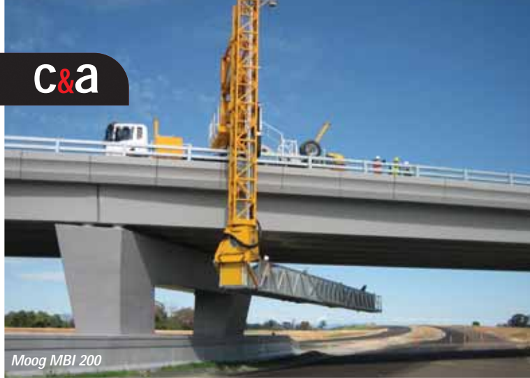
Moog gantries on the Soncutters Bridge in Hong Kong
