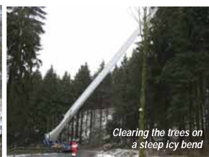
Raising the blade to clear overhead wires
