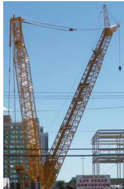
The 600 tonne Liebherr LR1600/2 will be one of the larger cranes on display
