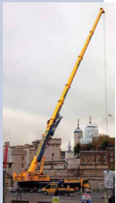
Three cranes were used in lifting various elements supporting the ice rink attraction in the dry moat beneath the Tower
