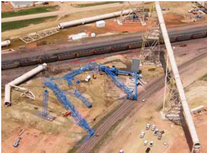
The large tube can that it was lifting can be seen on the left.
