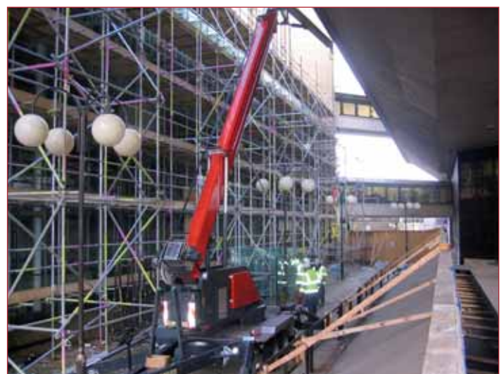
GGR was able to provide the Royal Bank of Scotland with a Skyworker crane after several other crane companies had to turn the job down. The Skyworker overcame restricted access problems and the need to reach over the top of the building to install the canopy glass.
