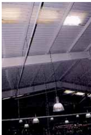
David Battisson fell 10m through this skylight into the store, which was open at the time.
