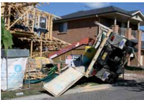
The majority of loader crane accidents are stabiliser related.
