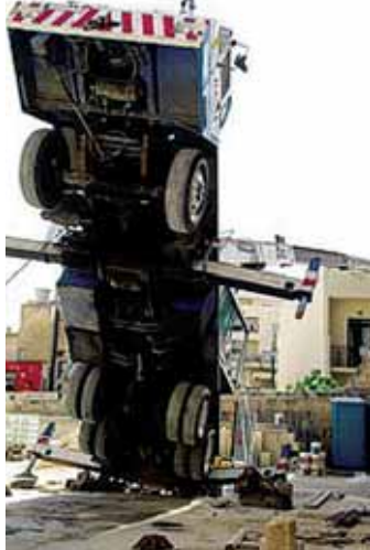
April 2007: A 40 tonne crane slipped off its home-made/make-do outrigger mats and tipped over in a street in Silema, Malta damaging buildings. Thankfully the operator was only slightly injured and no bystanders were involved.
