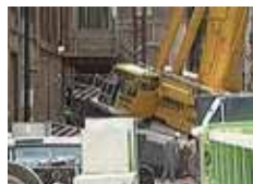
The 360 ton crane nearly ended up in the cellars and caused chaos in downtown Chicago.
