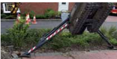
April 2007 Newbury, UK: An Italmec Ragno R16 was trimming trees when the edge of a loose bricked drive gave way resulting in the outriggers slipping off the drive causing the lift to tip, injuring
