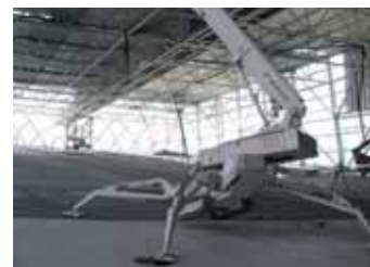
The Ommes were able to handle the 15° slope but used the non slip mats.
