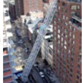
The main tower leans precariously against a building
